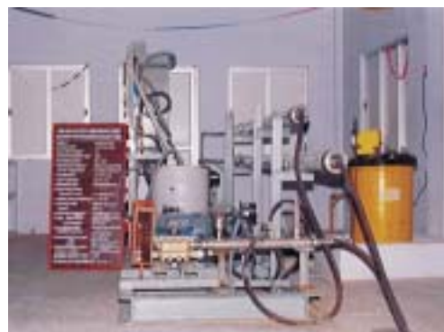
Photo 8.5: Reverse Osmosis Plant
